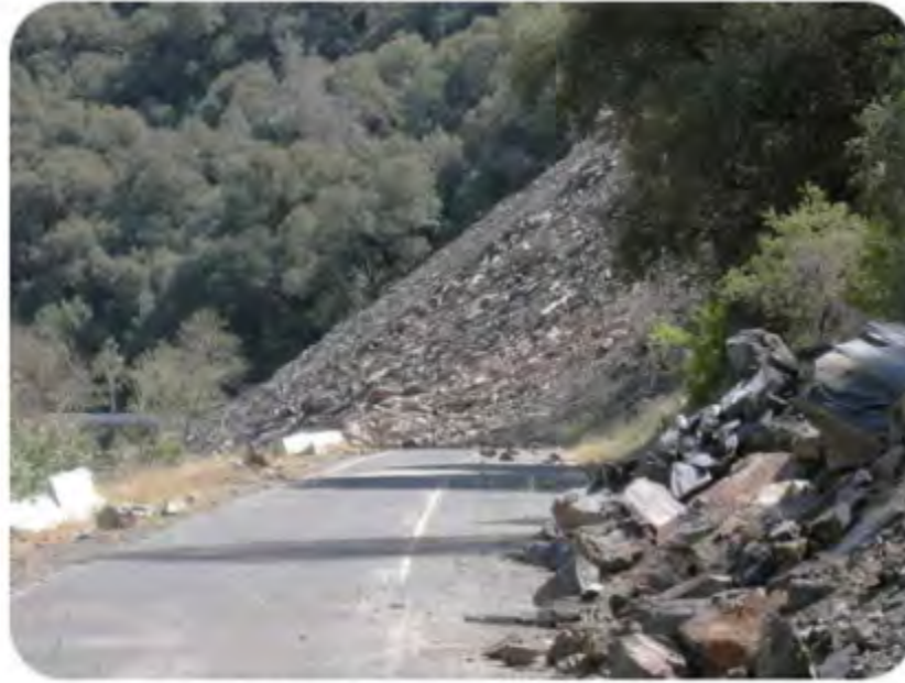
This landslide in California in 2008 blocked Highway 140. (ck12.org, CC BY-SA)
